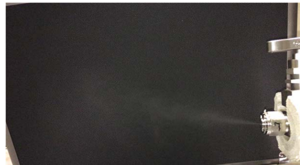
Fig. 3. Leaked steam through the crack
