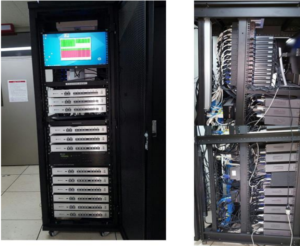
Figure 3 Validation Facility for display sharing function
