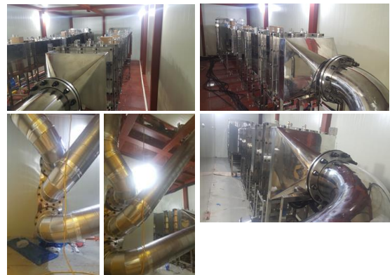
Fig. 3. Pictures of installed semi-plant facilities
