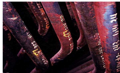
Fig. 5 Rusted feeder during normal operation
