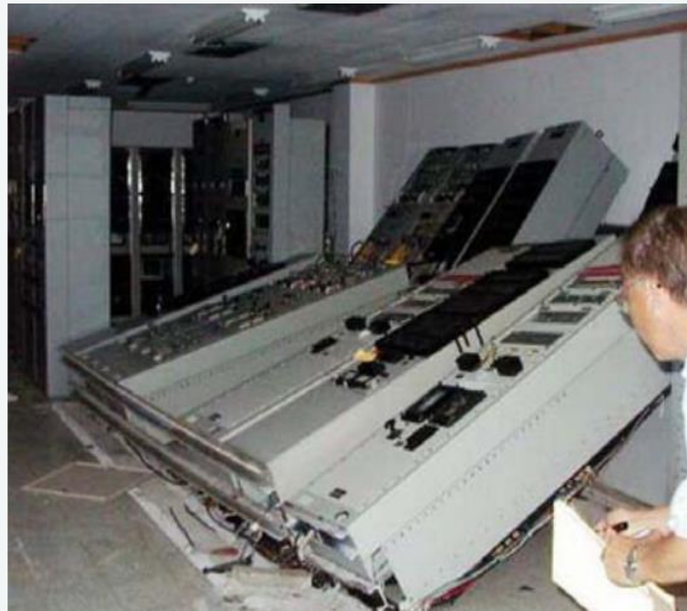
Seismic damage to anchored cabinets in 1985 Mexico Earthquake (Magnitude 8)
