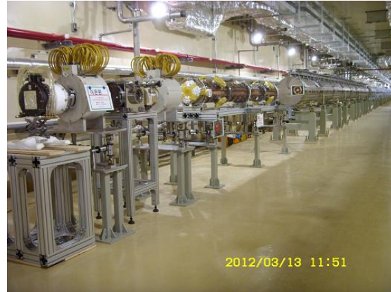
Fig. 6. 100MeV proton linear accelerator positioned in the tunnel from the injector to the beam dump.
