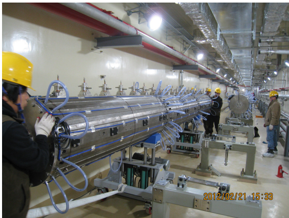
Fig. 5. DTL tanks were moved from the assembly area to the tunnel. Carriers and rollers were used.
