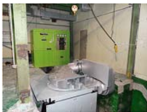
Fig. 4 Melting decontamination equipment
