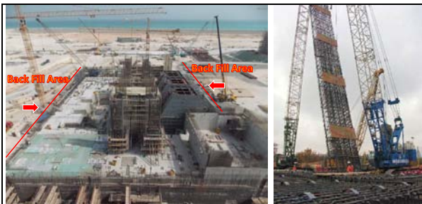
Fig. 13. Backfill area to use VHL crane around the TGB and lifting work of the pedestal column module.
