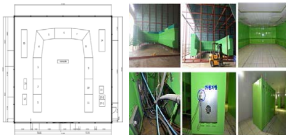
Fig. 1. Main control room and electric compartment installation
