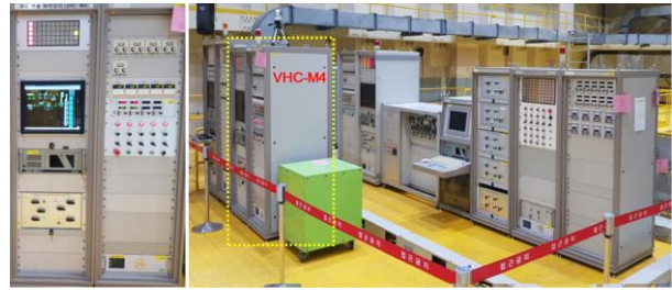
Fig. 5. A new capsule control system (VHC-M4) installed at HANARO
