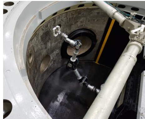
Fig. 1. The AURoRA robot installed in APR1400 Mockup.
