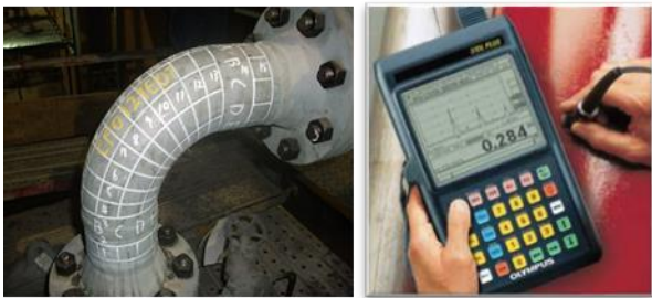
Fig. 1. Pipe wall thinning management in secondary systems of nuclear power plants using UT thickness inspection for mesh grids on piping components.
