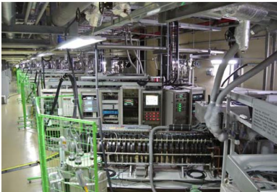
Fig. 1. Klystron gallery (klystron, circulator and LLRF system were installed in this place)
