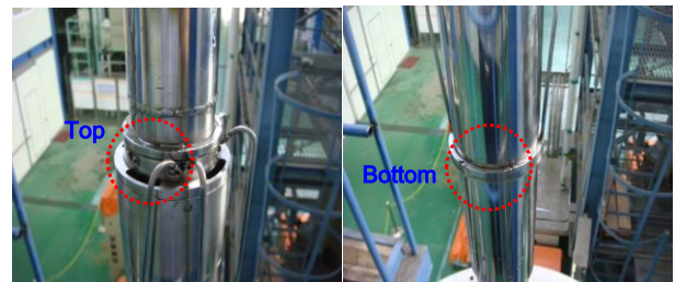
Fig. 4. The failure of the top guide spring during an out-pile testing of the long-term irradiation capsule
