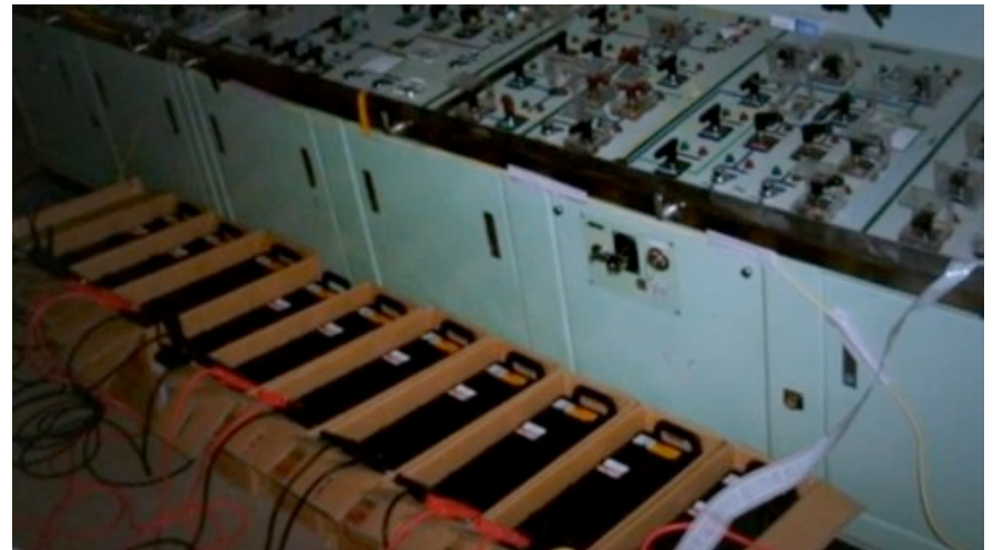
[Car batteries rigged together to power gauges]
