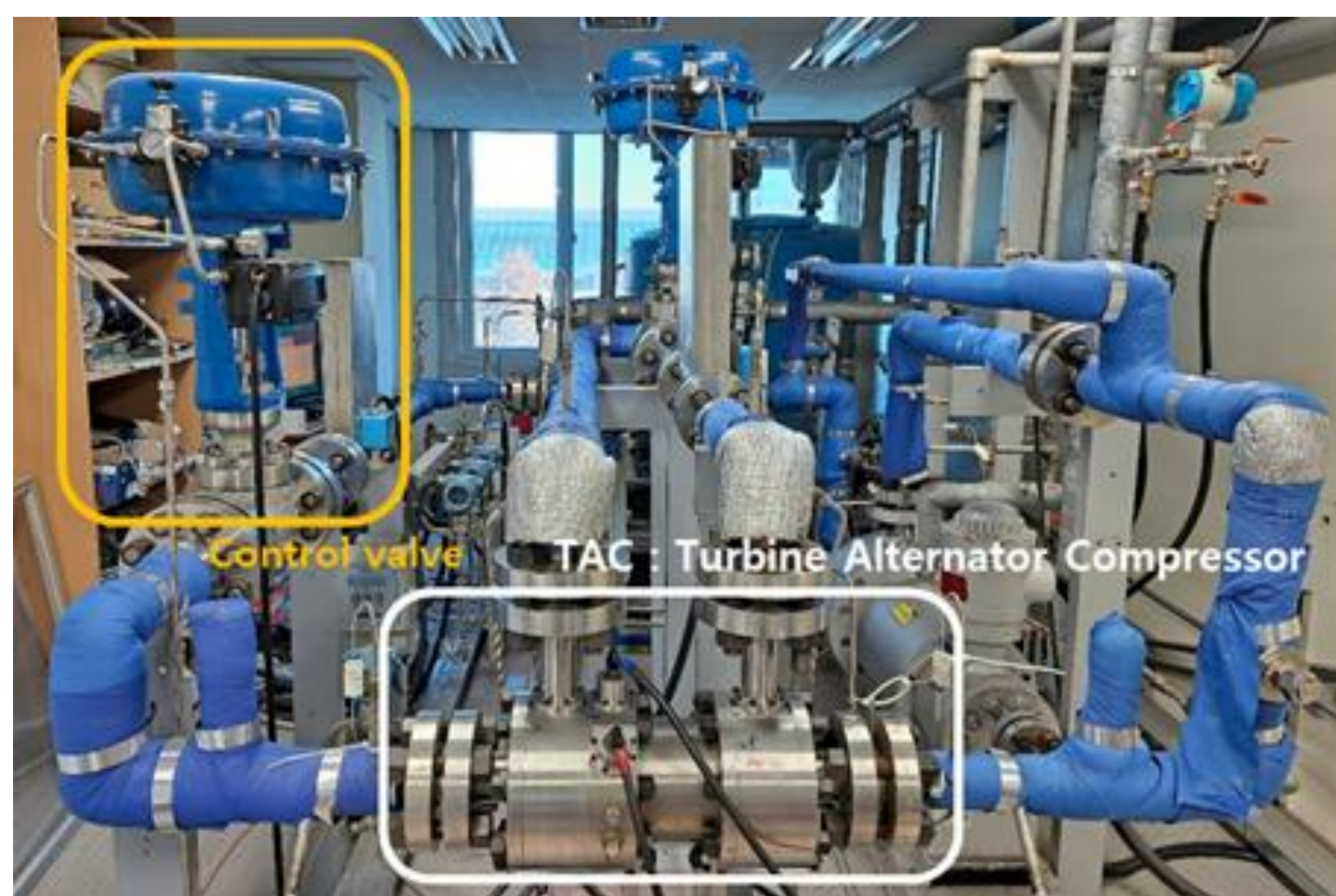
▲ Bird view of S-CO 2 compression test loop
