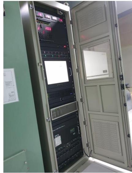
Fig. 2 The replaced seismic monitoring system in HANARO.
