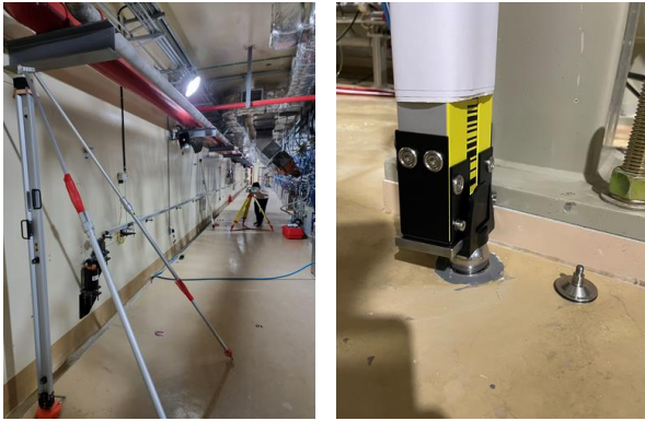
Fig. 4. Measuring the height of the ANs for the floor using a digital level
