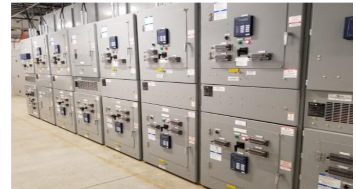
Medium Voltage Switchgear
