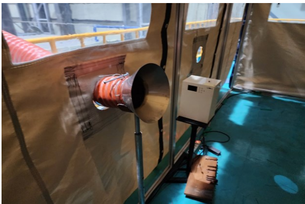
Fig. 3. Work tent equipped with mobile ACU inlet
