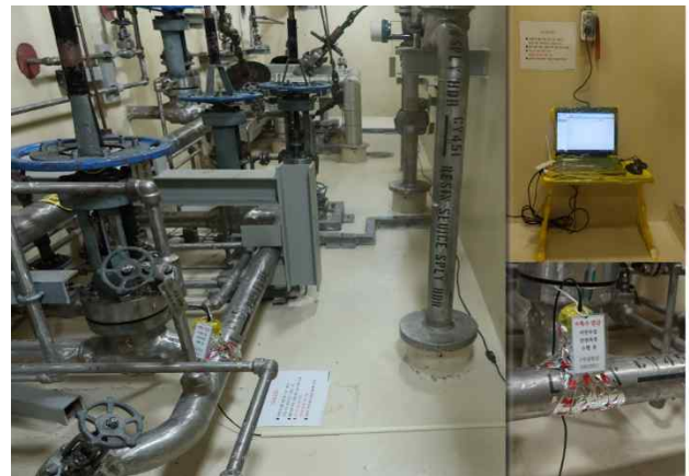
Figure 2. CZT install at the front of the CVCS filter
