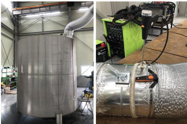
Fig. 2. An exhaust pipe installed in the manhole(left) and a hot wire anemometer installed in front of the damper, and NOx measuring device(right)
