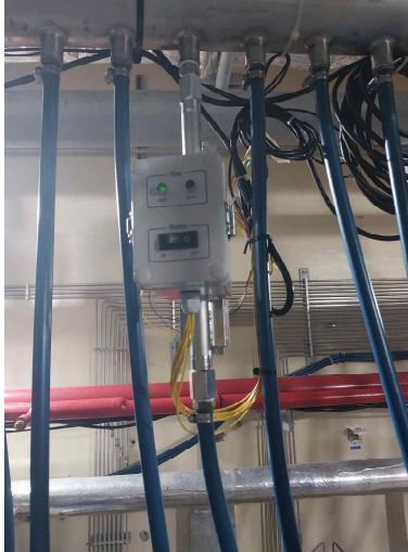
Fig. 9. Operation of the local monitoring box for the DTL 21 flow meter
