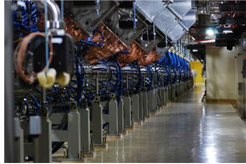
Fig. 2. DTL tanks at KOMAC
