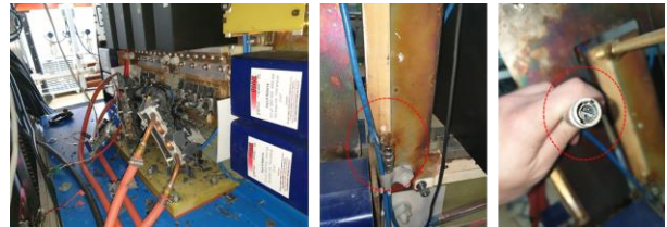
Figure 2 The IGBT blast (left) short between the high voltage line and Rogowski coil(right)
