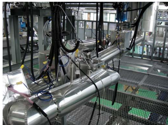
Fig. 3. Magnetic flow meter installed at the facility for instrument testing.
