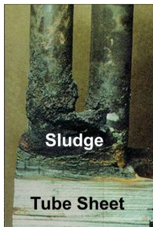
Fig. 1. Sludge pile above the top of tube sheet.
