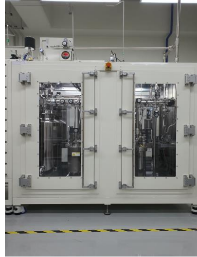
Fig. 3. Picture of Tritium Recovery System for Tritium Handling Facilities.
