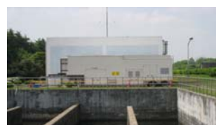
Fig. 2. Picture of installed MEB at site.
