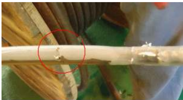
Fig. 4. A hole in cable insulation of specimen no. 6
