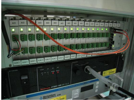
Fig. 3. Analog transition converter installed on high voltage platform
