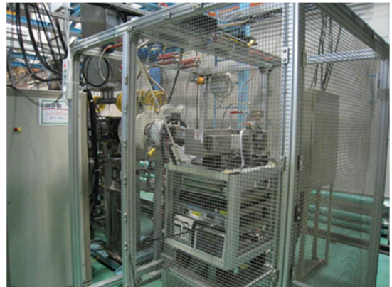
Fig. 2. Microwave ion source installed in 20-MeV proton linac
