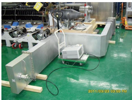
Fig. 5: The fabricated penetration waveguide
