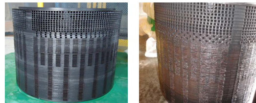
Fig. 1. Photos before and after the EFCV Cage clogging of YGN #5 and #6
