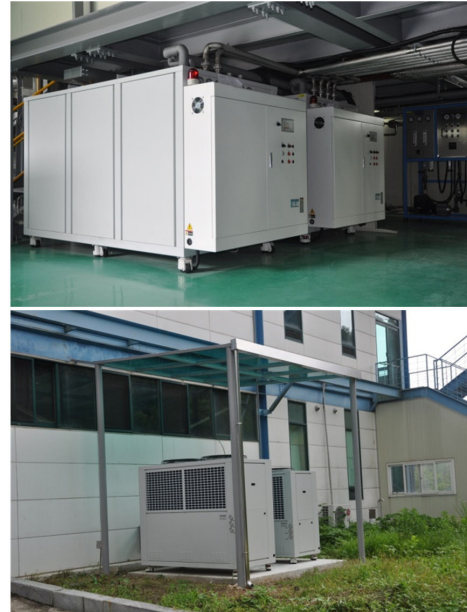
Figure 5. Photo of chiller system
