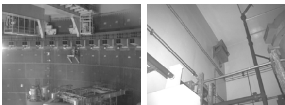
Fig. 2. PARs installed high level in Shin-Kori-1 and in Kori-1 containments. Caution should be used for the access.
