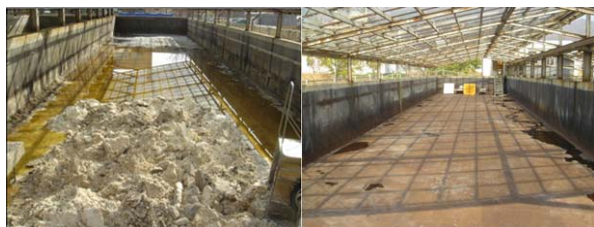
Fig.4. View of lagoon before and after sludge waste treatment
