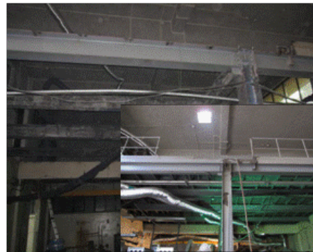
Fig.2. Before and after dismantling of the steel structure in the AUC process region
