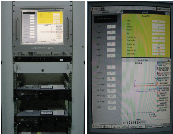
Figure 2. The channel access gateway of the PEFP control network.
