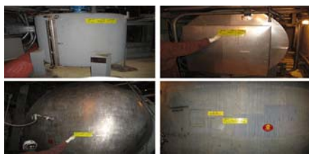
Figure 4. Tanks inside Containment Building
