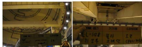
Figure 2. Polar Crane located at Upper Side of Containment Building of Yonggwang Unit 1&2
