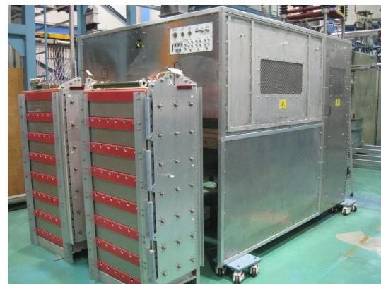
Fig. 8: Tank assembly and capacitor bank
