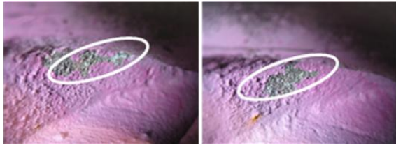
Fig. 4 Picture of paint wears of impeller vane tip and the middle of vane (in the white circle)
