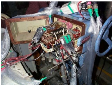
Fig 1: A picture of installed sensors at a field test
